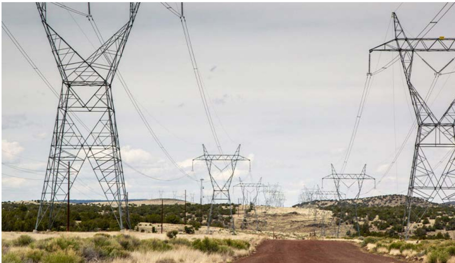
Transmission lines in WAPA's Desert Southwest Region | Western Area Power Administration
