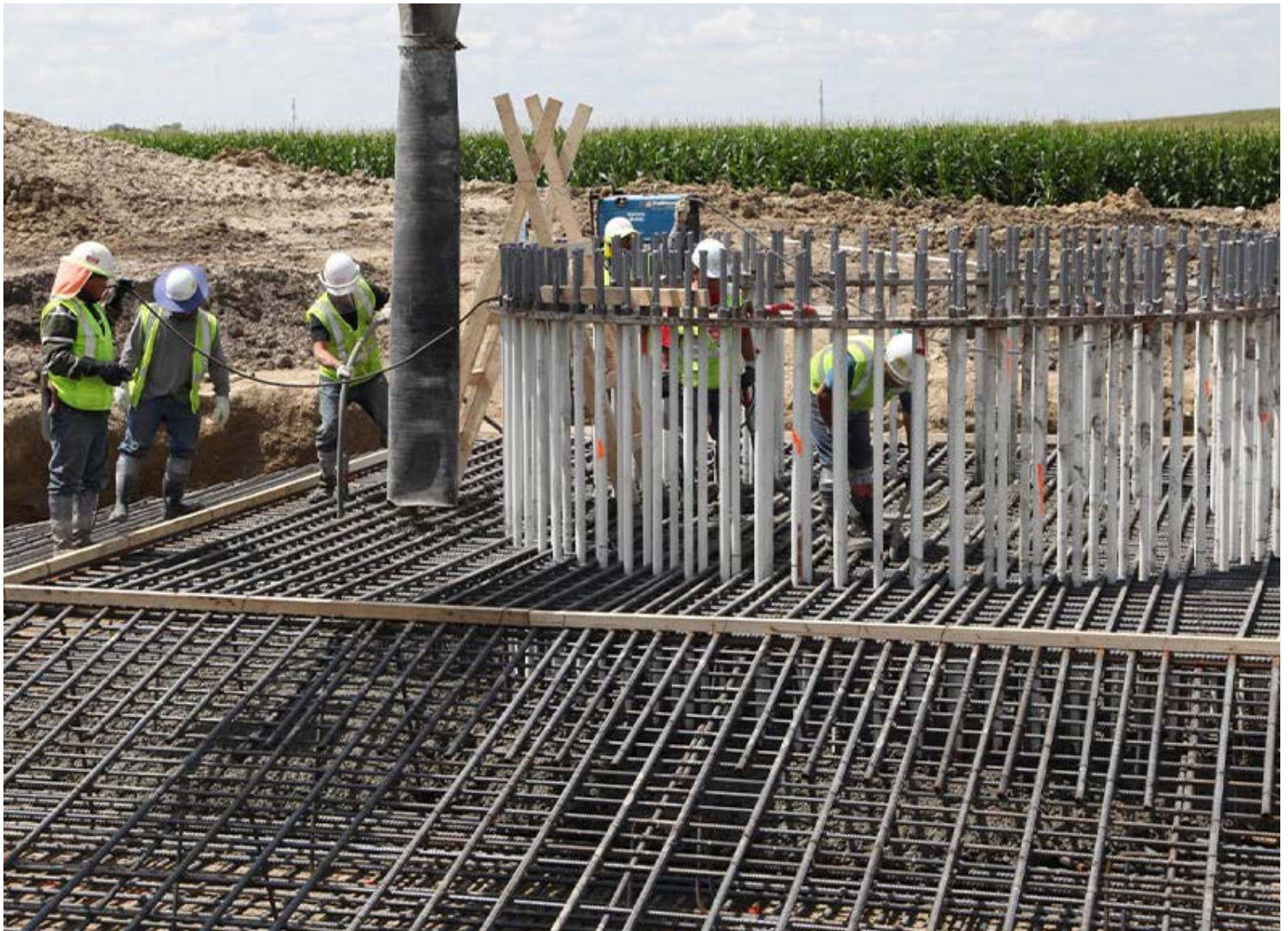
The Fagen Civil Crew pours the first wind turbine foundation at the Palmer's Creek Wind Farm project in Minnesota in 2018. The wind farm's network upgrade agreement was among those filed unexecuted in protest over MISO's reinstating transmission owners' right to self-fund network upgrades. | Fagen, Inc.
